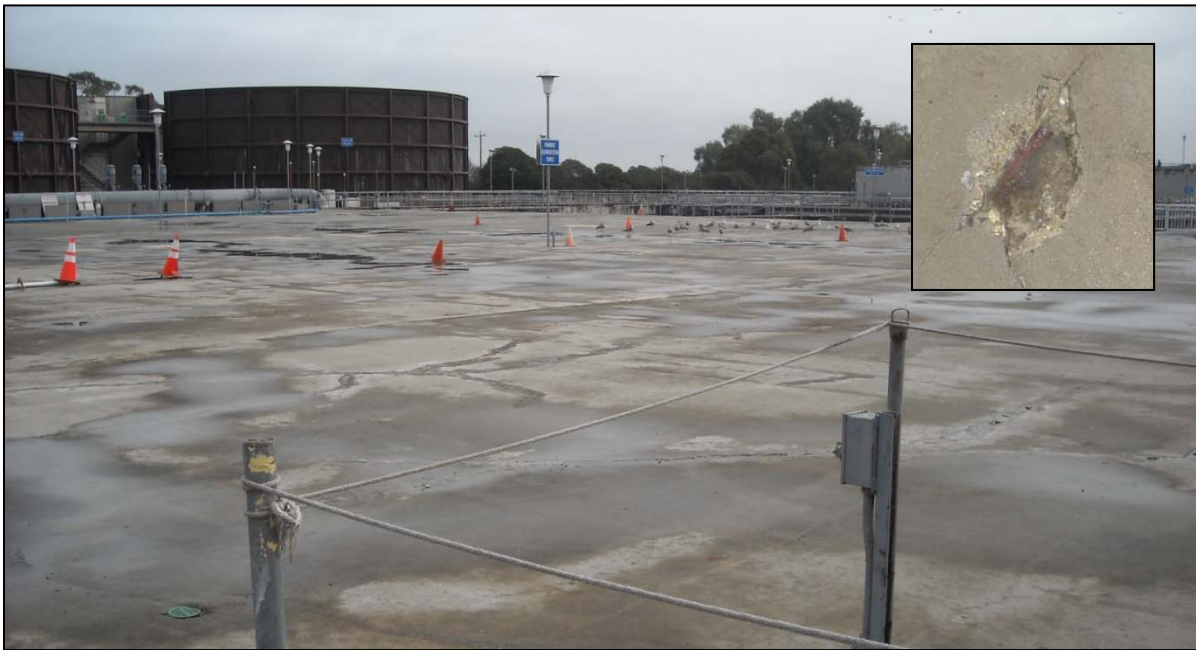
Figure 5.2 Cracks Observed on the Primary Sedimentation Tanks Roof
