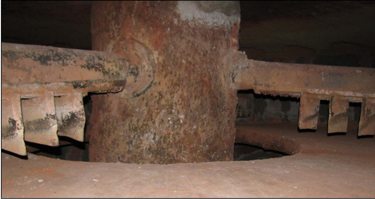
Figure 5.5 Corrosion Inside the Hearths of the Multiple Hearth Furnaces
