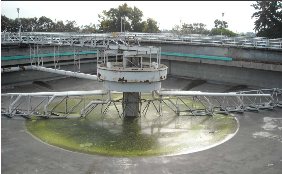
Figure 5.4 Visible Corrosion on the Secondary Clarifier Equipment
