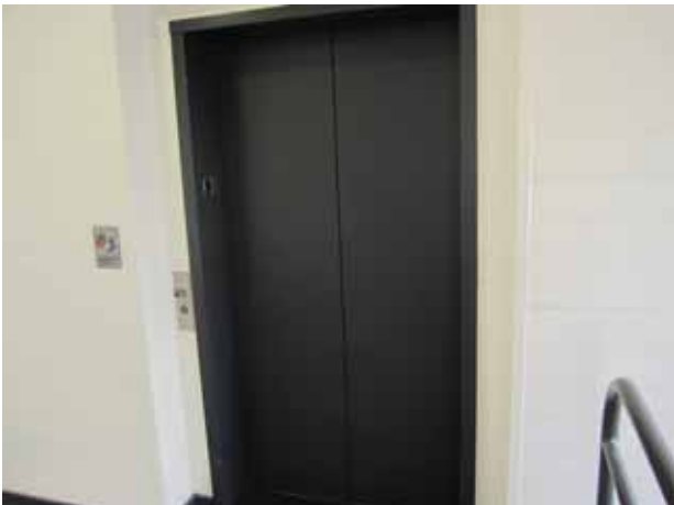
17. View of a typical hydraulic elevator located inside the subject property building.
