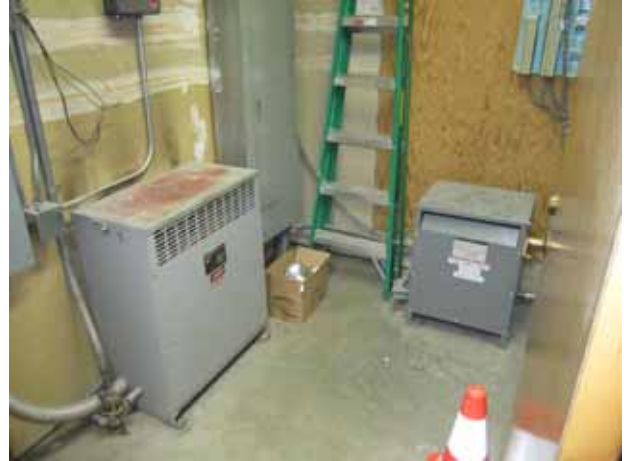
20. View of typical interior transformers located inside the subject property building.
