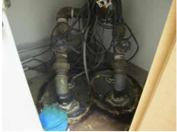
32. View of the dual sump pump at the kitchenette located inside the Suite A-20 onsite.
