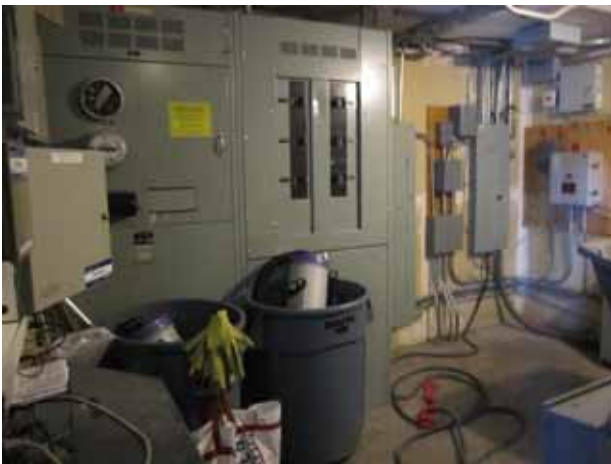
21. View of the main electrical room located inside the subject property building.
