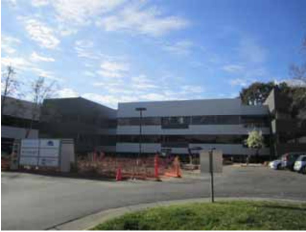
13. View of an area under construction, located at the central portion of the subject property.
