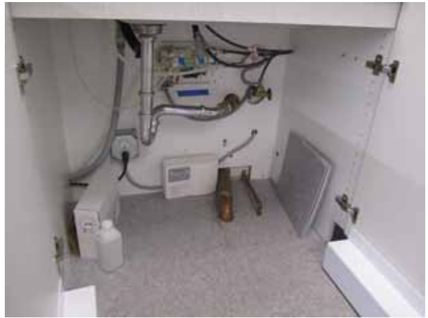
28. View of a typical under-the-counter, tank-less water heater located inside the building onsite.
