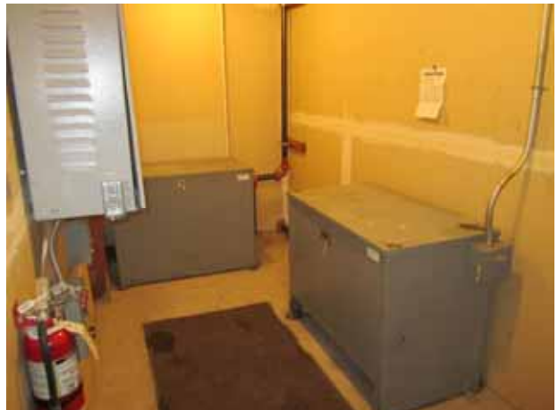
18. View of the hydraulic elevator equipment room located inside the subject property building.
