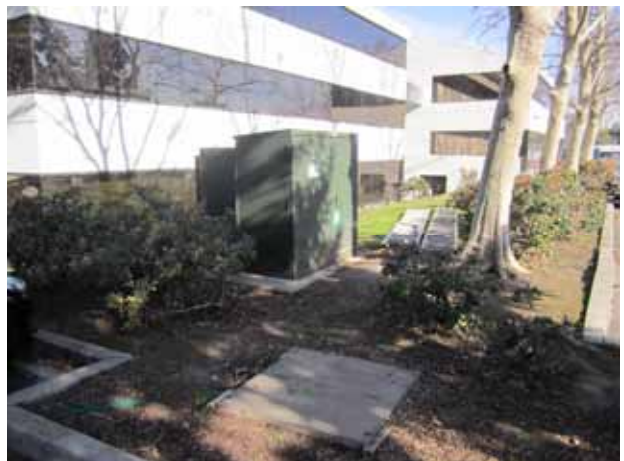
6. View of the transformer located adjacent to the southeast of the subject property building.
