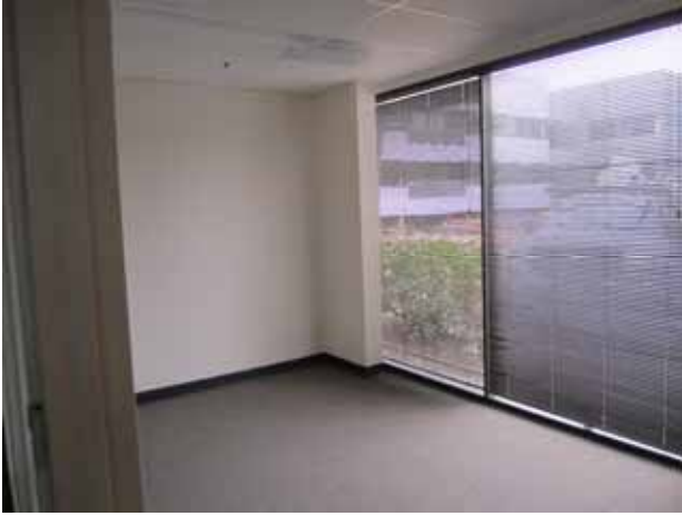
25. View of the general office space located inside the vacant Suite A-24 at the subject property.
