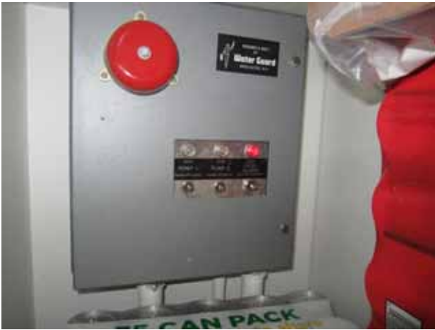
33. View of the controls for the dual sump pump at the kitchenette located inside the Suite A-20.
