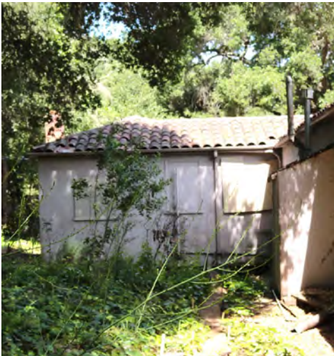
Figure 11: South-facing wall of 1928 addition. Looking north. Source: Halsey House HSR by ARG, taken in May 2019.
