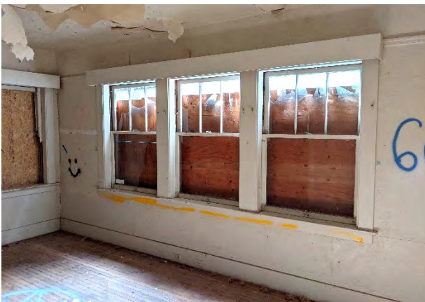
Figure 14: Interior view of three grouped typical double-hung windows along south façade of west wing. Looking southeast.
