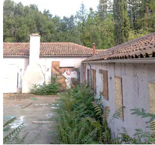
Figure 19: North and east sides of rear courtyard (south- and west-facing wall). Looking north over rear courtyard wall.
