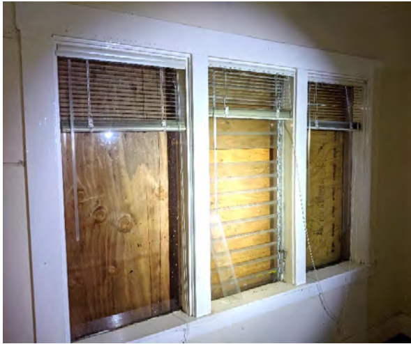
Figure 8: Interior view of jalousie and fixed windows along primary façade. Looking northeast.
