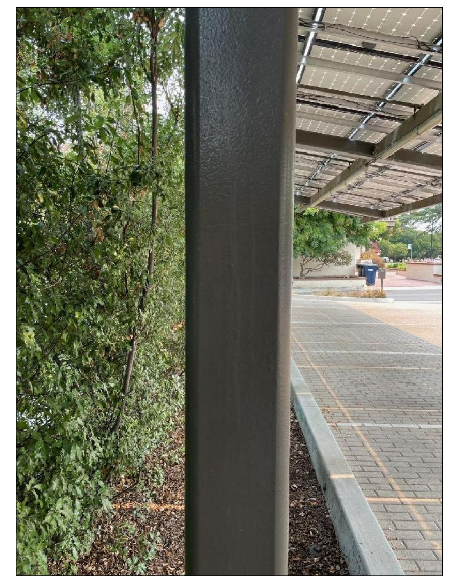
EXISTING PACKARD FOUNDATION PARKING LOT AT 323 2ND STREET: RECTANGULAR STEEL TUBE COLUMN
