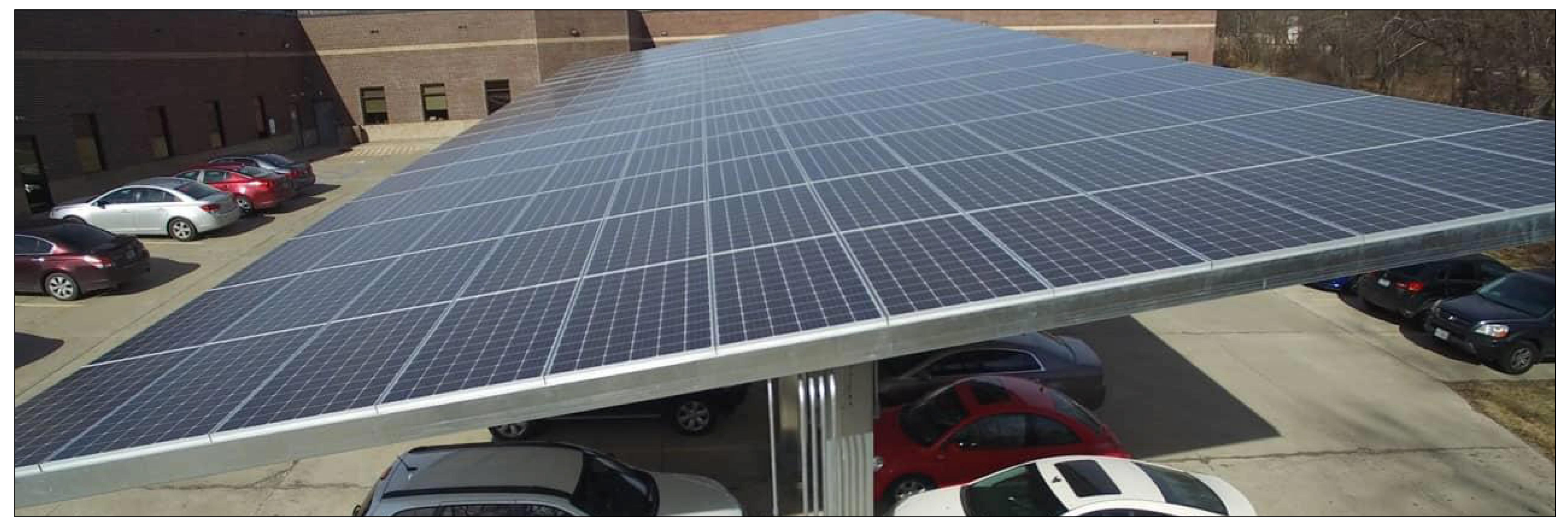
SHALLOW PITCH ROOF WITH FLUSH MOUNTED PV PANELS
