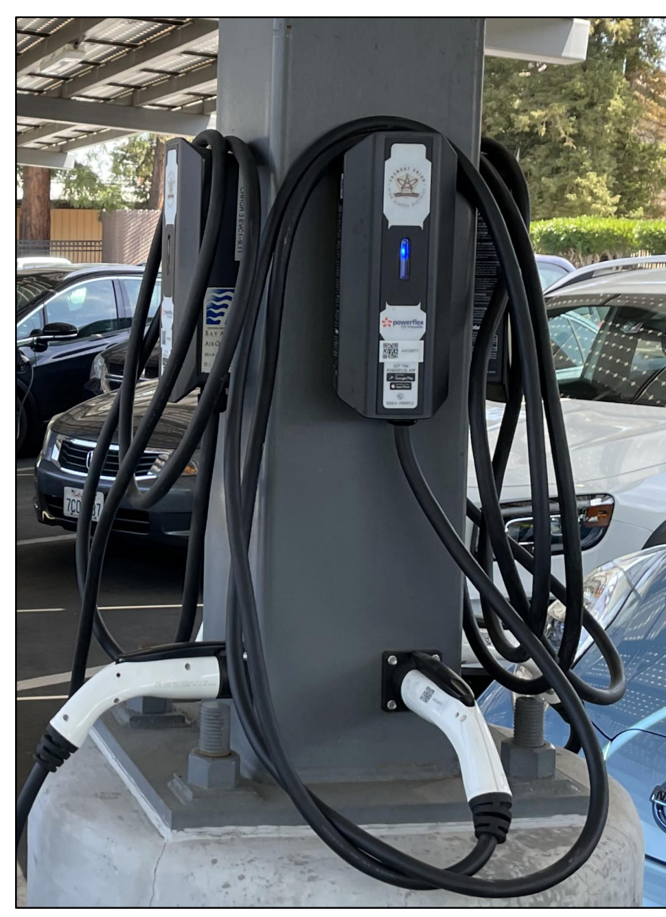
EV CHARGER COLUMN MOUNTED
