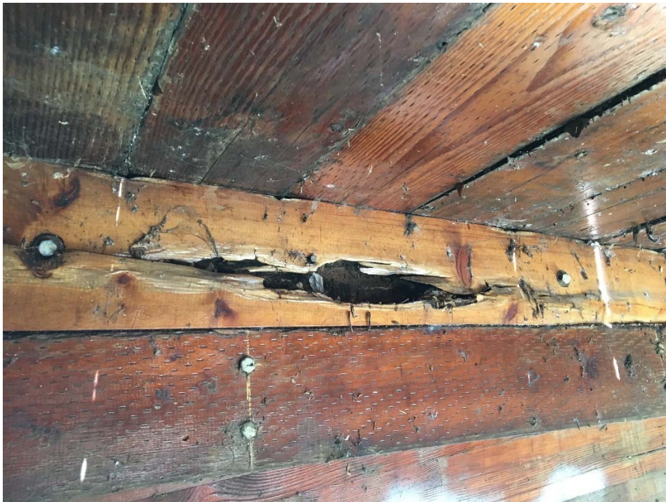
Figure 4 - Pedestrian Bridge blocking with severe deterioration
