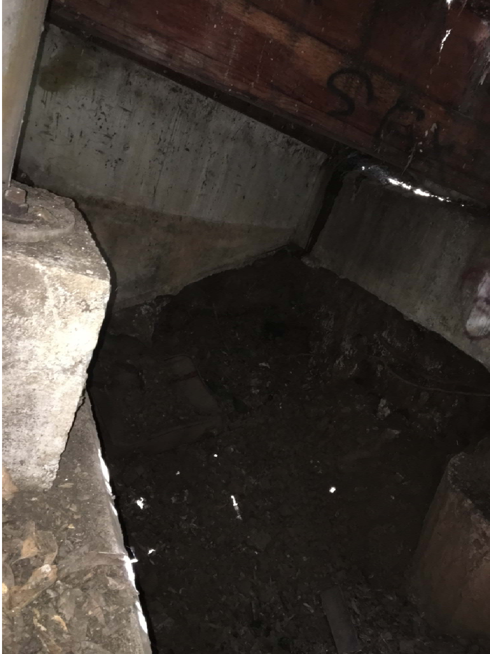
Figure 8 - Pedestrian Bridge bin abutment with scour
