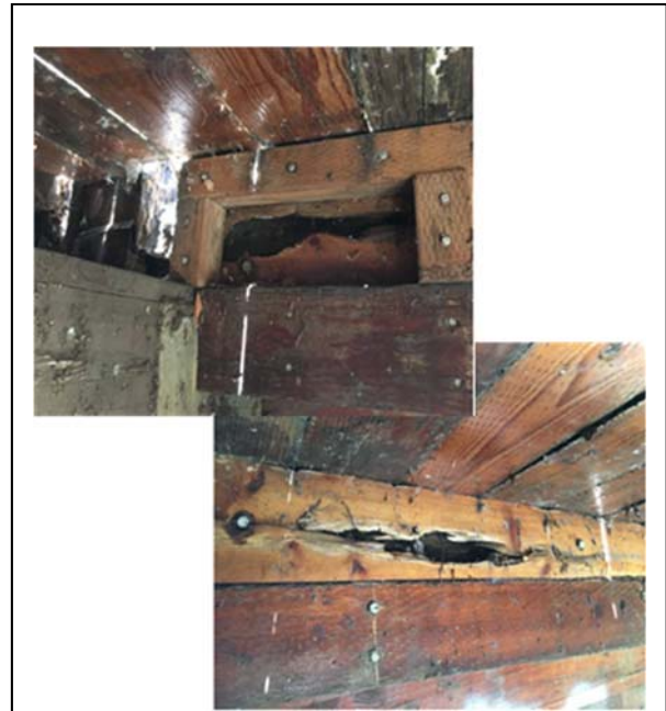
Figure 3 – Structural Blocking Dry Rot
