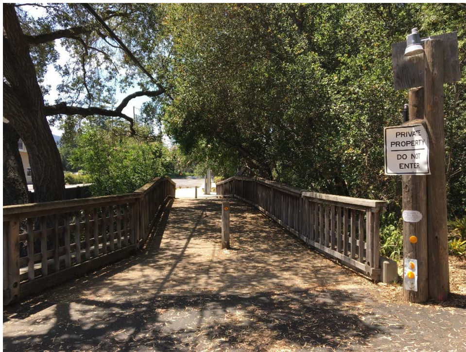
Figure 2 - Pedestrian Bridge looking west with close proximity to trees and overhead utility
