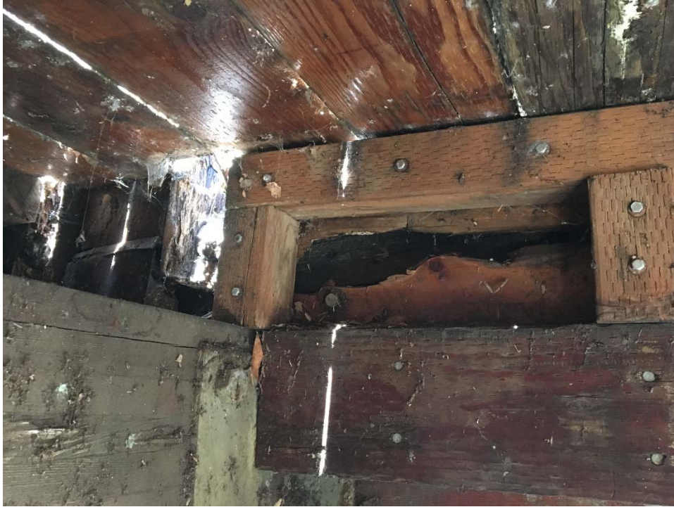
Figure 5 - Soffit of Pedestrian Bridge with blocking and handrail post deterioration and repaired section
