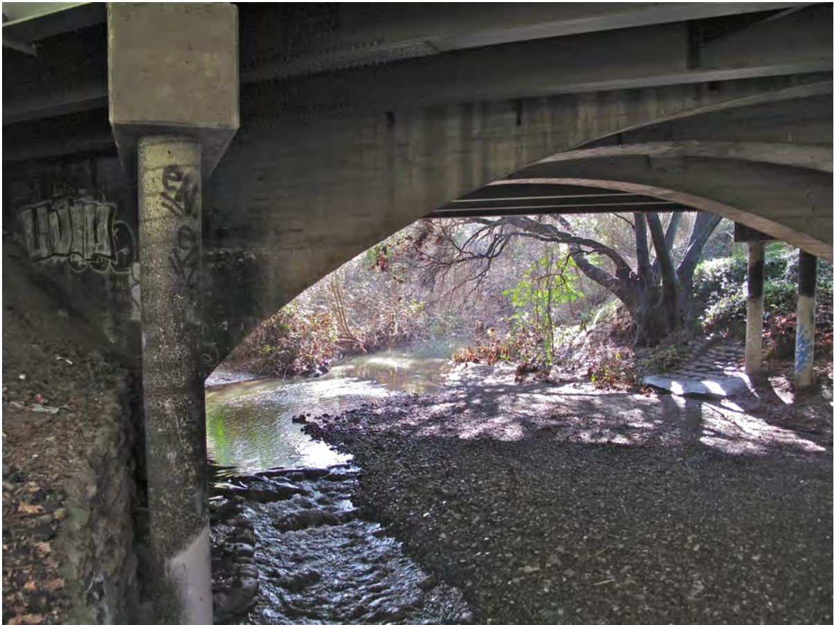
The concrete arch bridge that spans Stevens Creek at Fremont Avenue cannot be modified to accommodate a trail underpass.
