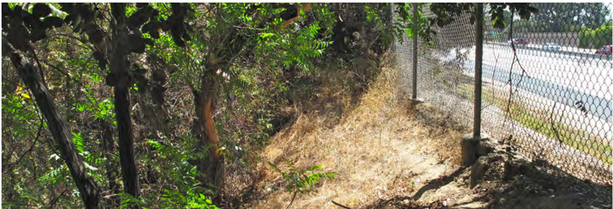
Inadequate Top-of-Bank south of the SCVWD Fremont Drop Structure adjacent to State Route 85.
